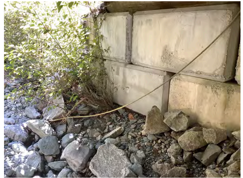
Missing riprap - woods side downstream
